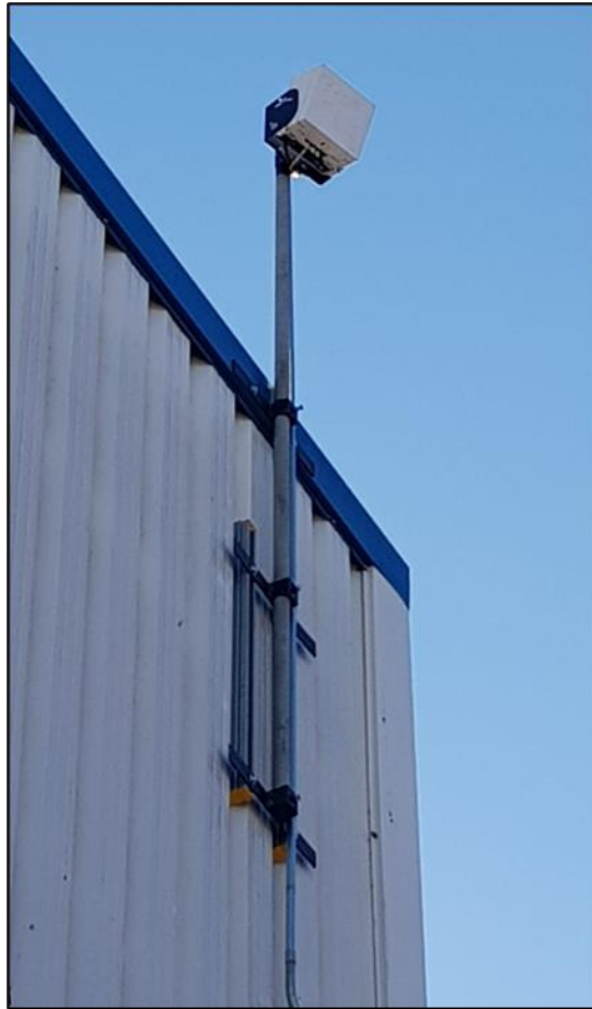
Figure 14: Outdoor antenna installed at SP-ExFa (Ford)
