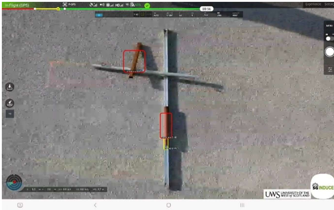
Figure 40 Corrosion detection of different pipes with areas non-corroded.
