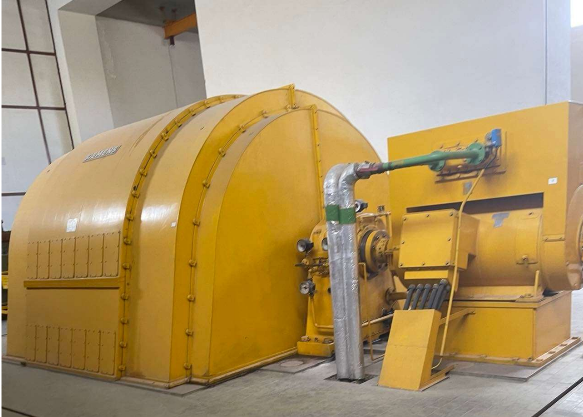
Figure 33 Power Generator at PPC premises used in UC4.
